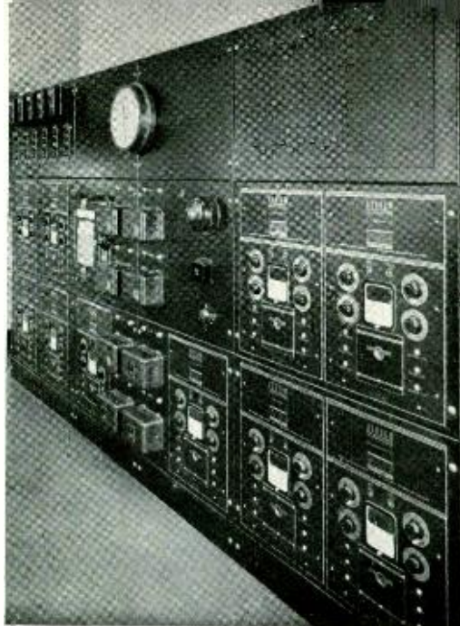
On a board behind the desk in the control center is the supervisory equipment for heating, ventilating and power supply
