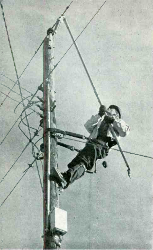
A lineman uses a "hot stick" to connect a coupler for high-frequency telephone carrier
