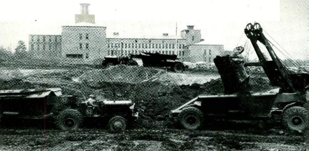
Excavating in preparation for the addition to the Murray Hill buildings which is now under construction and which will more than double their present size
