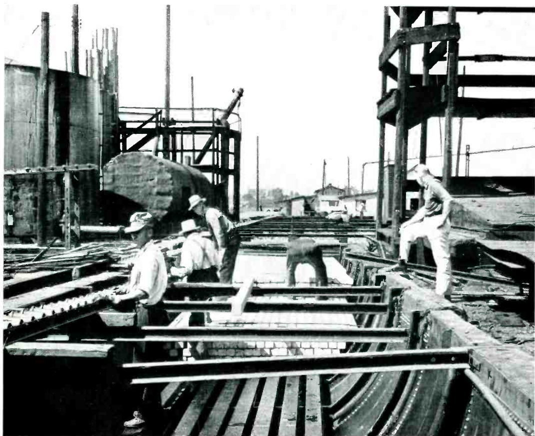
Fig. 2—Steel rails are used to counteract the buoyancy of the arms in the preservative. R. H. Colley supervises the stacking of the crossarms in the treating tank at St. Paul
