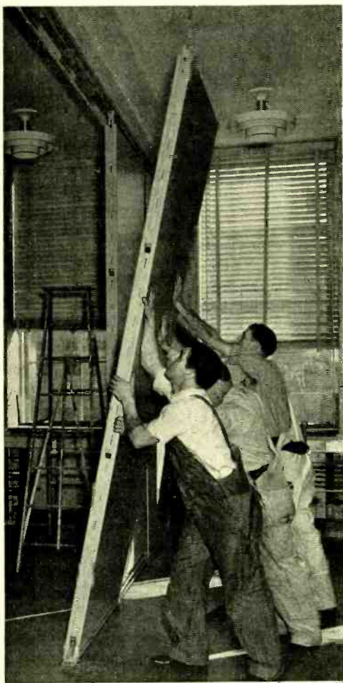
Fig. 2—Placing one of the steel panels in position in the Murray Hill Laboratories
