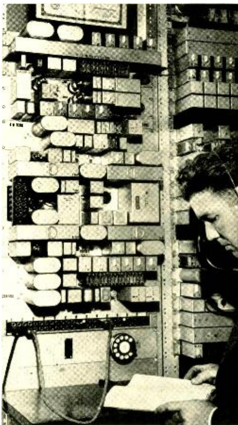
Fig. 5—Terminal bay at the Crisfield office
