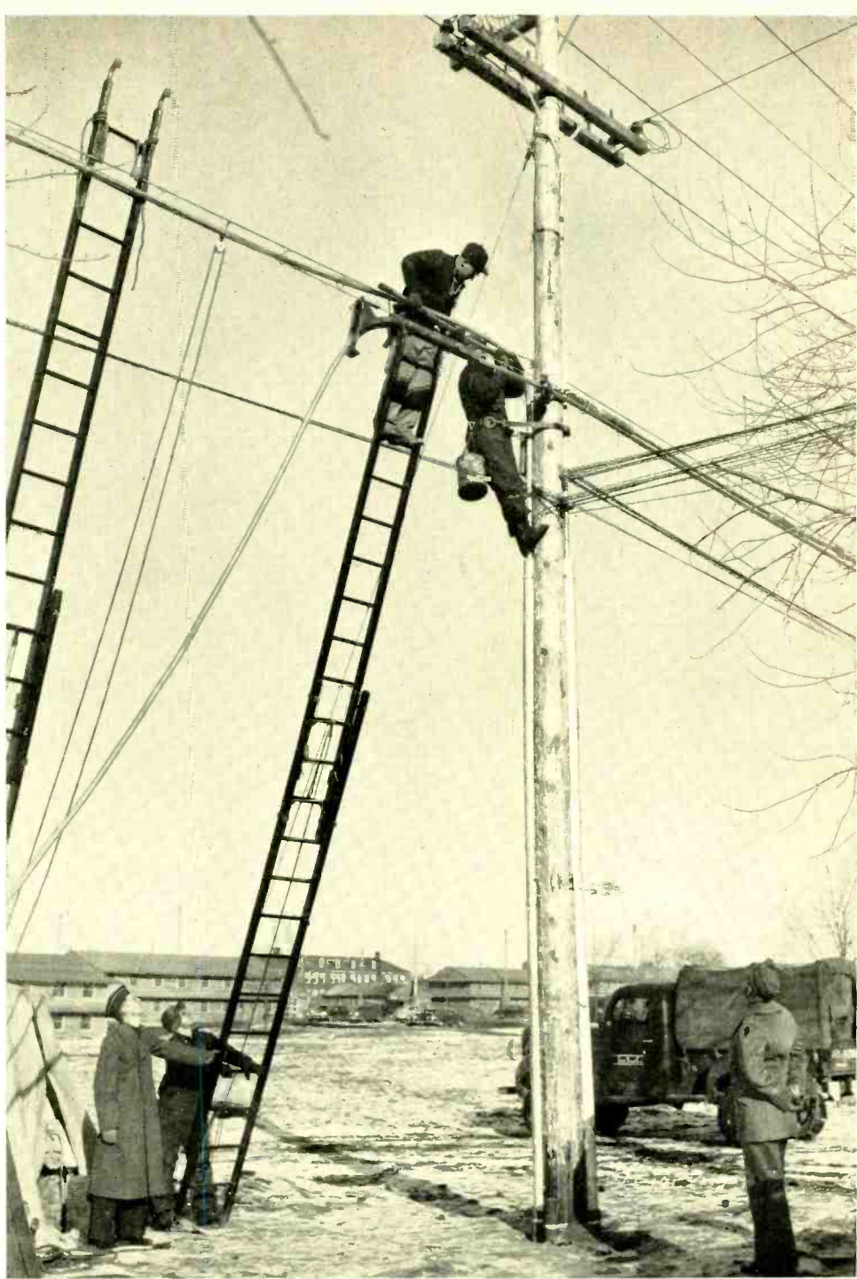
At Fort Custer, near Battle Creek, a Michi- gan Bell crew installs new 303-pair cable
