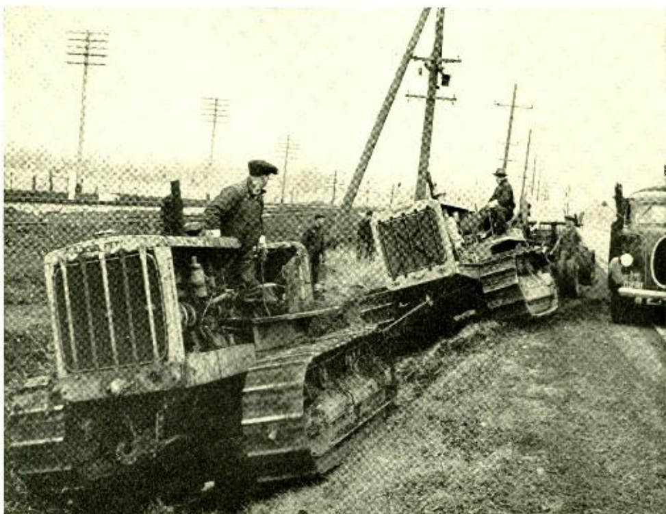
To clear the open-wire telephone lines from a large area where a munitions works is to be erected, the Illinois Bell Telephone Company has transferred a number of its important circuits to a cable shown here in the process of being laid by a buried-cable train
