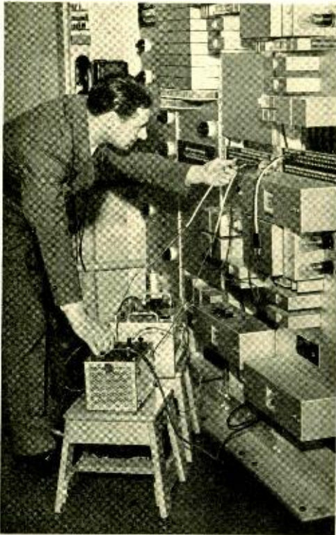
Fig. 5—Making a transmission test on one of the repeaters used for the demonstration toll call at the New York World's Fair. Three circuits are available: one in use, and two serving as spares. Each circuit has a repeater and a group of associated equipment. In addition there is a bridging amplifier that is used to supply the receivers for the visitors to the exhibit
