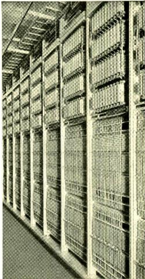
Fig. 1—Block relay bays, each with forty block relays above, and line cross-connecting terminals for their NC and NF leads below
