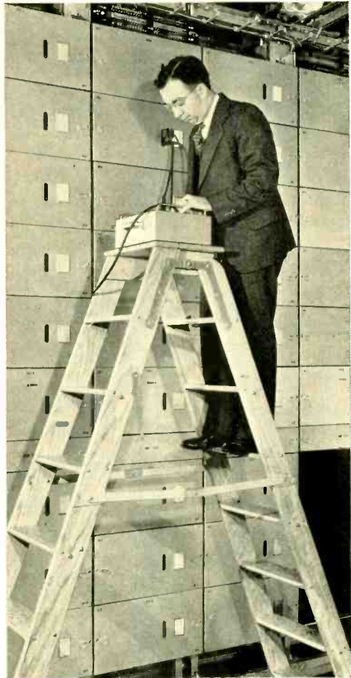
Fig. 1—Portable set being used to test vacuum tubes of type-K amplifiers in the Long Lines building in New York City
