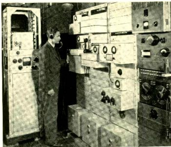
Fig. 9—Modulating terminal equipment at the New York end of the coaxial circuit
