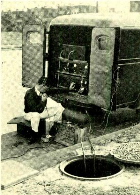
Fig. 6—A field test being made of the coaxial cable after it was installed
