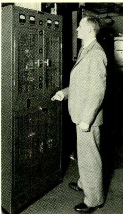
Fig. 2—The new 100-watt transmitter, known as the 15A, makes small demands on space and is simple to operate
