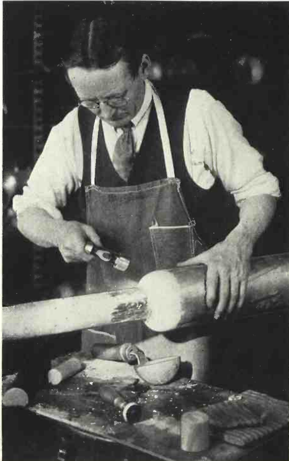
Fig. 1—After the sleeve has been slid over the splice its ends are beaten down into contact with the cable
