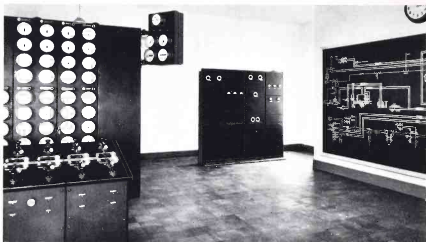
Fig. 5—Carrier terminal equipment in the control room of the Newark Substation
