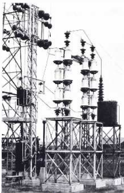
Fig. 2—110,000 volt coupling equipment at Station "J"
