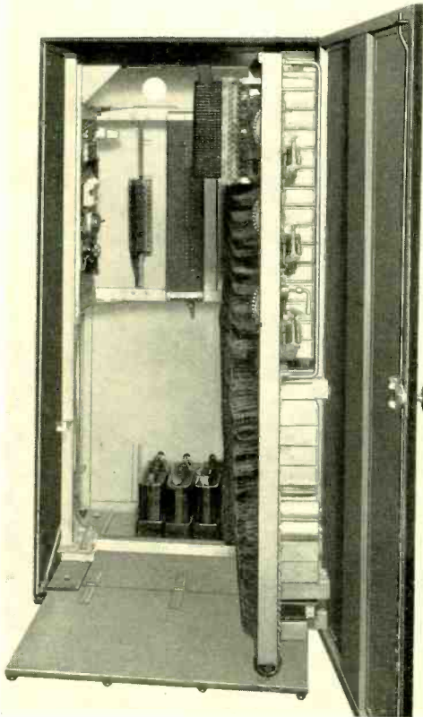
Fig. 4—Complete accessibility to the wiring and apparatus was obtained by mounting the switching equipment on a swinging gate
