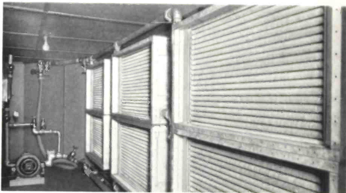
The radiators and pump
