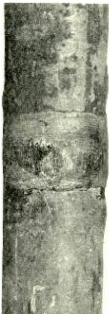
Factory joint in 1887 cable. Present cables are covered by a continuous sheath
