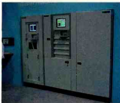
Comark will supply Advantage and DCX IOT tube-type transmitters and Ultimate and Optimum solid-state units.
