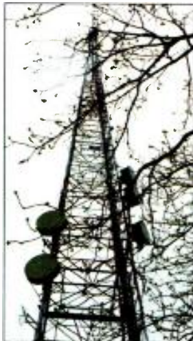
WETA-TV's DTV broadcast antenna shares a tower with WETA-FM in suburban Washington
