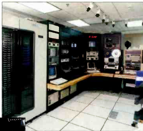
Communications Engineering Inc. completed this new digital origination facility for BET Jazz.
