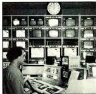
NBC's Olympics control room
