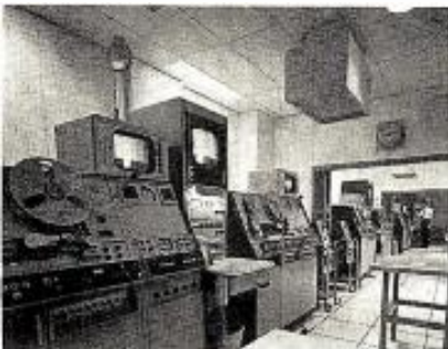
The video-tape array in the production center includes eight Ampex VTR 2000's and two Ampex VTR 1200's. Four of the machines are equipped for electronic editing. There are also slow-motion machines.
