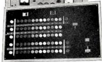
Typical Control Panel
