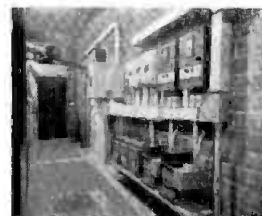
Layout of wall-mounted switchgear. Heavy components are installed at floor level which eliminates need for reinforcing the tile wall.
