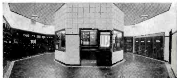
The BTA-50G occupies less than 15 feet of wall space, as seen at the right. At the left, a portion of the old composite 50 KW transmitter can be seen which takes up approximately 2½ times as much wall space, as the Ampliphase Transmitter.
