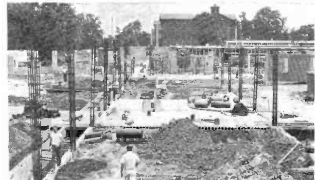
A MUCH NEEDED LARGE ADDITION now under construction at Longview State Hospital.
