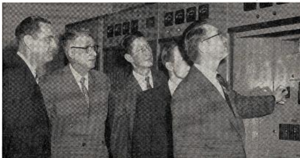
WTAR Norfolk, Va., has put in operation a new $22,000 am transmitter with a new $6,000 auxiliary, both features of a $1 million expansion program which brought improved facilities to WTAR and its sister stations, WTAR-FM and WTAR-TV. Making a final check are (l to r) John Pepper, assistant general manager; Campbell Arnoux, general manager; Bob Lambe, general sales manager, Jack Black, radio sales manager, and Dick Lindell, chief engineer.
