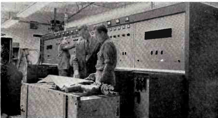
G-E field engineers Stone, Bias and Duncan (l. to r.) work on the installation of the first 12-kw transmitter built by G.E. for WHUM-TV.
