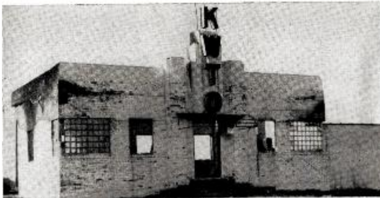
← KWTO transmitter building looked like this after fire.
