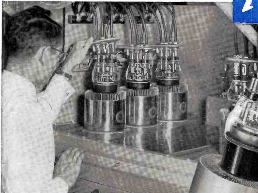
Installation of Federal F-8C25 power triodes in modulator tube compartment of 207B-1 transmitter.
