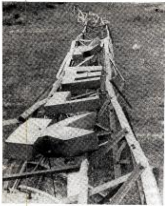
TOWER of KELK Elko, Nev., looked like this after an 80-mile-an-hour gale hit it last month. Van Welch, station's chief engineer, reports KELK was back on air with temporary antenna less than 10 hours after tower went down. KELK is erecting new 200-ft. permanent tower. Station operates with 250 w unlimited on 1340 kc.
