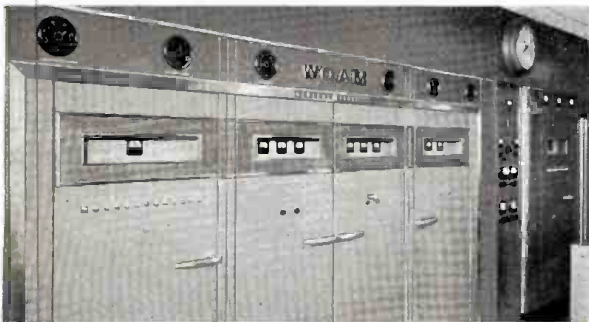
WQAM—MIAMI —The clear, strong signal from this station blankets greater Miami and gives dependable coverage of the 15 additional counties in its trading area. Above: G-E 5 kw AM transmitter. (left), Monitor rack, G-E 10 kw FM transmitter (background).
