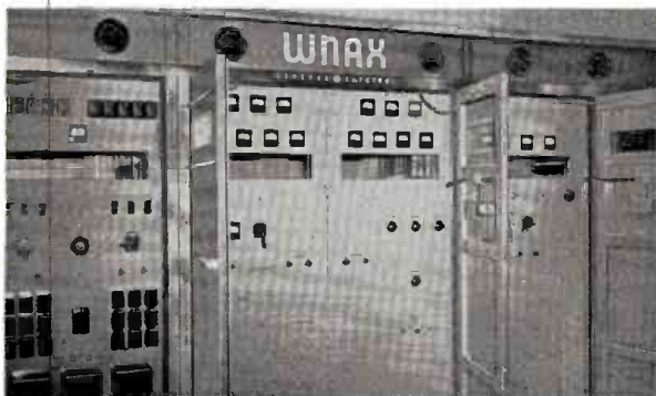
WNAX—YANKTON —A Cowles station, on the air since 1926. This South Dakota station recently modernized its broadcast facilities, installing a General Electric 5 kw AM transmitter.
