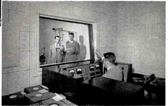
The new master console in the control room, from which point engineers channel the daily flow of network and local programs. All new equipment embodies the latest developments in radio engineering.
