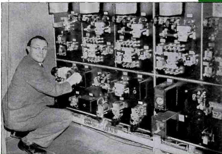
JOE WHITEHOUSE , Chief Transmitter Engineer, makes an adjustment on the largest relay panel ever employed by any commercial radio station in the United States. This relay panel, created in the WLW research laboratory, operates a transmitter line throughout the transmitter.
