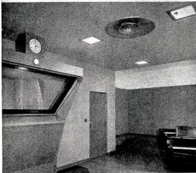
To meet today's exacting standards for high fidelity broadcasting, this studio utilizes the USG system of Sound Control
