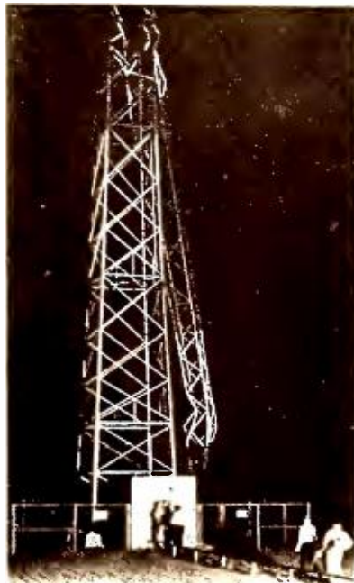
AFTER THE STORM—The tower of WSPD looked like this after it was struck by a terrific windstorm.
