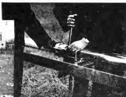
Below: A view of the installed line leading from the transmitter to WTAM's tuning tower.
