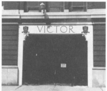
Figure 4. Front door view of Building #17, with "VICTOR" engraved in the masonry over the door.
