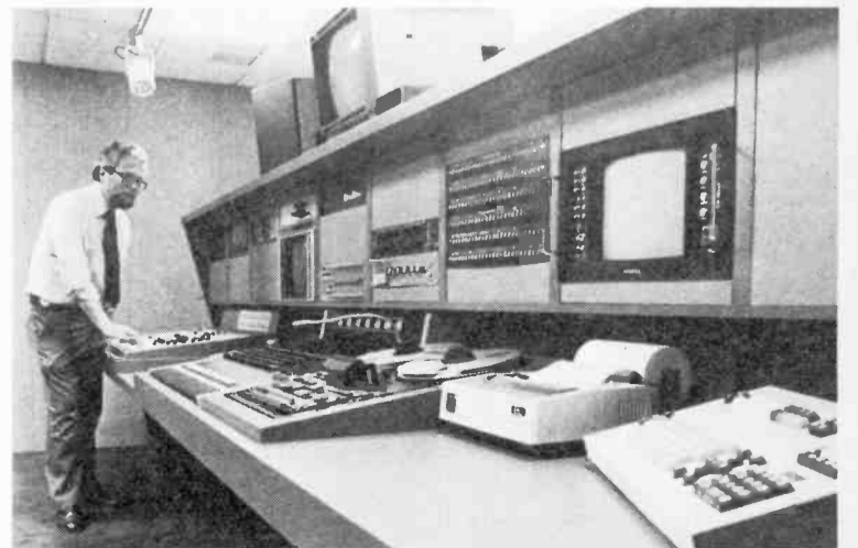
TESTING, TESTING —Walter Rauffer, Movielab Video vice president of engineering, checks newly installed equipment in the post-production facilities. Left to right are a Grass Valley switcher, CMX editor, Audioarts mixing console and Chyron IV character generator.
