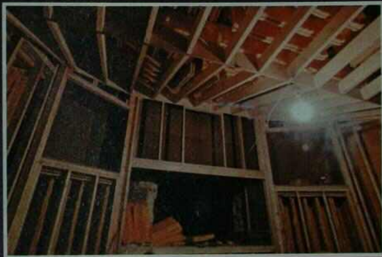
Structural View of One of the Quad Control Rooms
