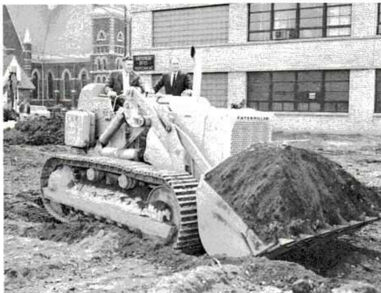
BALLY PRESIDENT BILL O'DONNELL takes the controls of the big Cat to break ground for the company's new 20,000-square-foot addition to its plant on Belmont Avenue on Chicago's North Side. Engineering and manufacturing facilities will be housed in the addition. Also pictured above is Bally sales manager, Paul Calamari.
