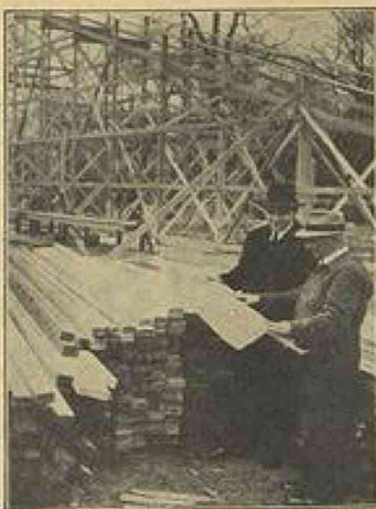
RIVERSIDE PARK, Springfield, Mass., having announced a $50,000 expansion program for its second year of operation, Edward J. Carroll (left), owner-manager, is seen here going over plans with Joe Drambour, new Coaster contractor, with construction under way.
