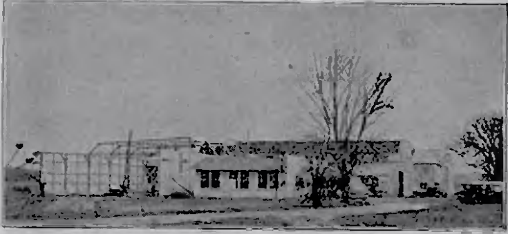
THIS SALEM, ORE., SCENE SHOWS the original plant and the new addition under construction by the Eperly Aircraft Corporation. This annex is to be the assembly shop for the Loop-o-Plane and Octopus rides produced by this firm.
