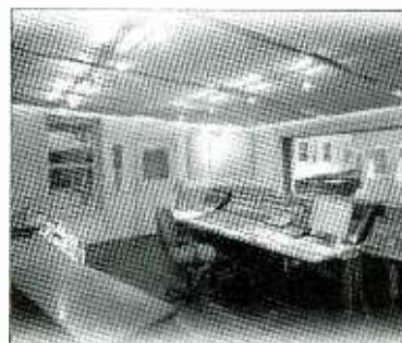
Clubhouse Headquarters. The control room at the Clubhouse features a Neve 8058 Mk II console.
