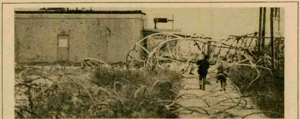
TOWER TUMBLED — Severe winter winds toppled the 2000-ft. KWWL-TV/Waterloo, IA tower, knocking KFMW/Waterloo off the air for more than a week. Above, two KWWL-TV staffers view the damage, which will take 9-12 months to repair.
