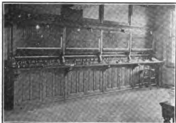
VIEW OF THE SWITCHBOARD.
