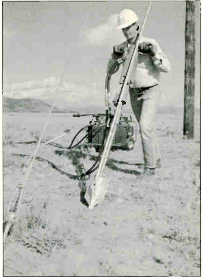
Drive type anchors are driven into the ground by one or two men using a jackhammer.
