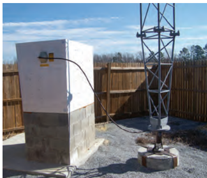
High-Power Antenna Tuning Units
