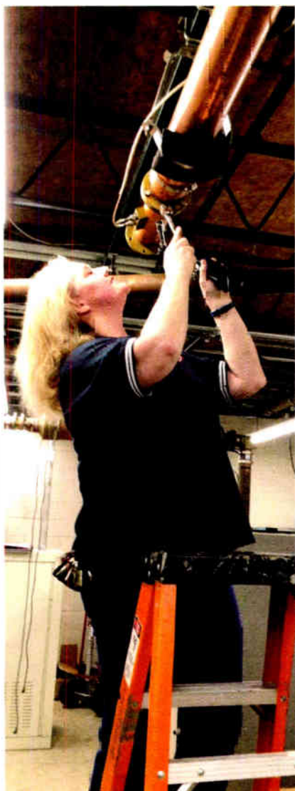
Sherri Powers is shown at the main transmitter site for WDMK and backup of WMGC. The staff nicknamed the site "Gotham." Powers was replumbing the old WDMK transmitter to feed the WMGC antenna.
