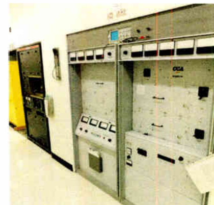
WWV 10 MHz transmitter and standby.
