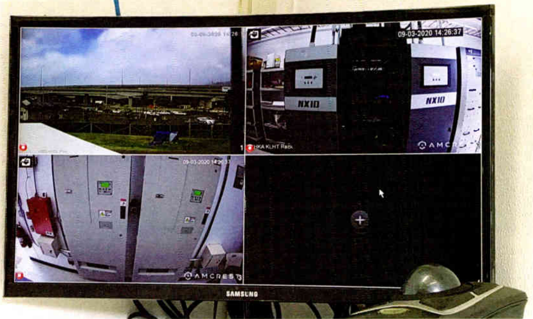
Fig. 6: Compile a screen to show both inside and outside the transmitter site.
