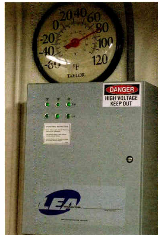
Fig. 4: How about checking your Surge Suppression status, before arriving at the site?
