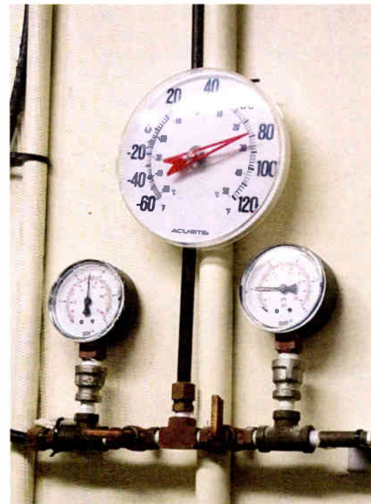
Fig. 3: Pan in another direction to check the room temperature and N2 pressures.
